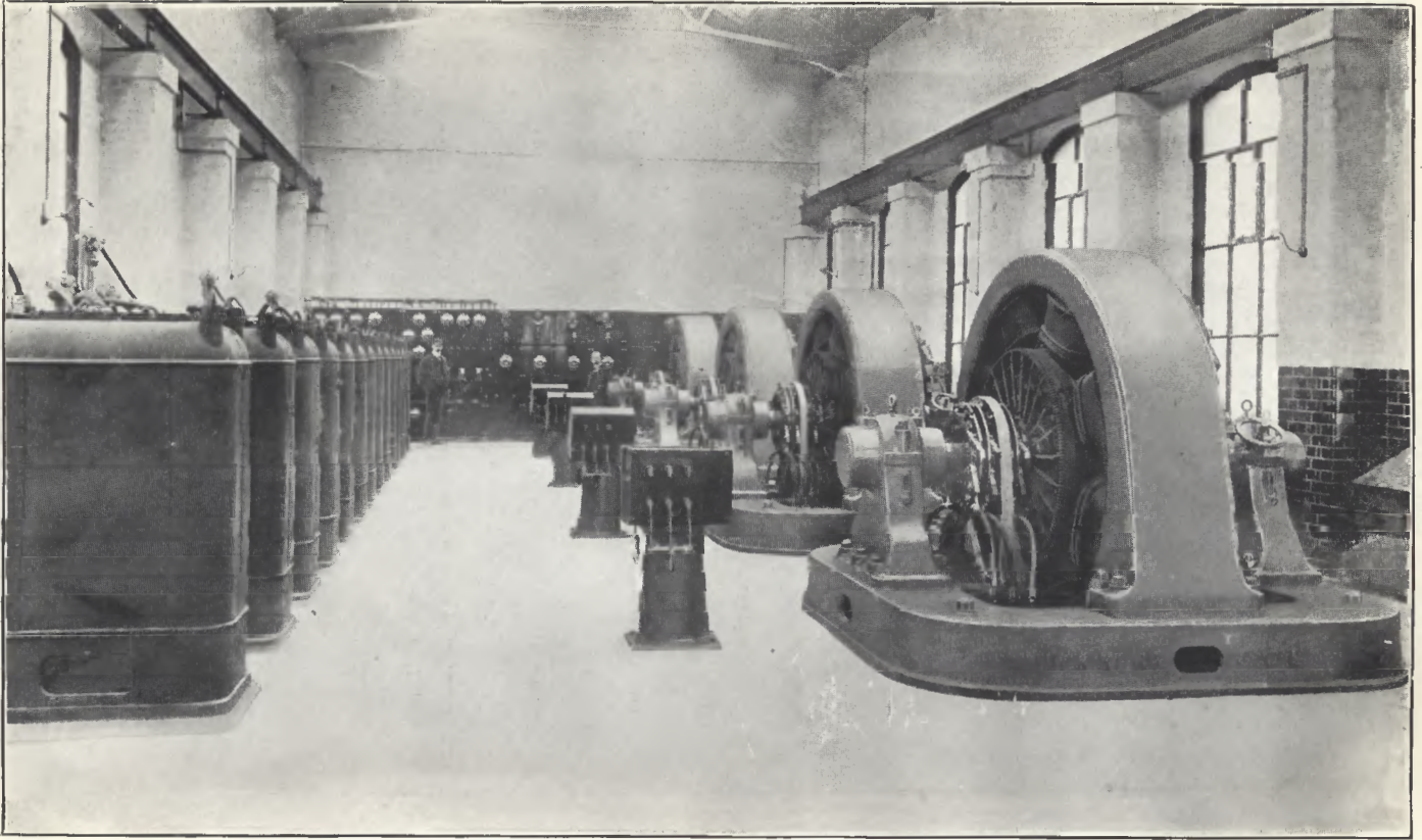
INTERIOR OF SUB-STATION.
